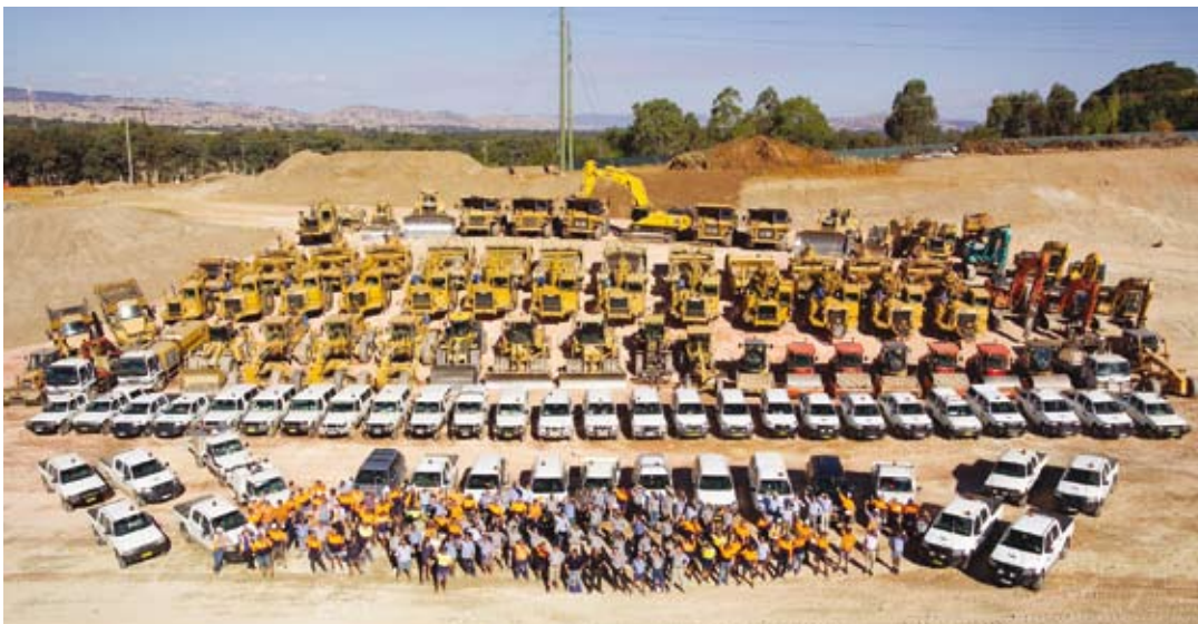
Figure 5.9 – Part of the fleet used during the construction phase in Abigroup’s $383 million Albury Wodonga Hume Freeway project between 2005 and 2007
